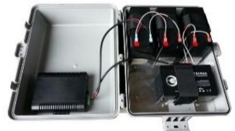
10A Solar, 30W PoE Controller Inside
