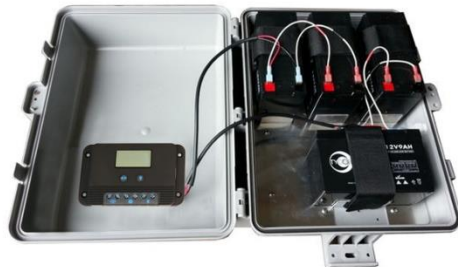
20A PWM Controller Inside
